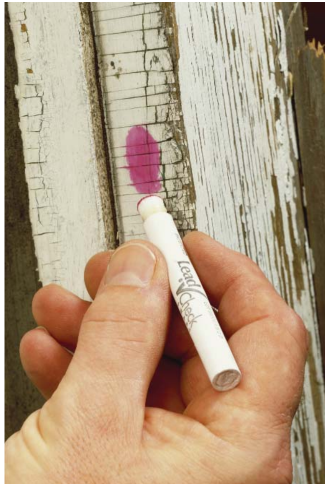
A swab test shows this painted surface is positive for lead.
