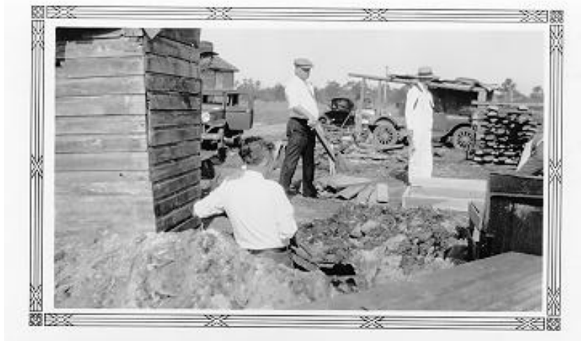
Figure 13. Using Works Progress Administration (WPA) funds to construct privies in the mid 1930's – Source: Florida Department of Health Photo Archives.
